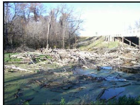
decaying tree debris impairs water quality and threatens infrastructure
