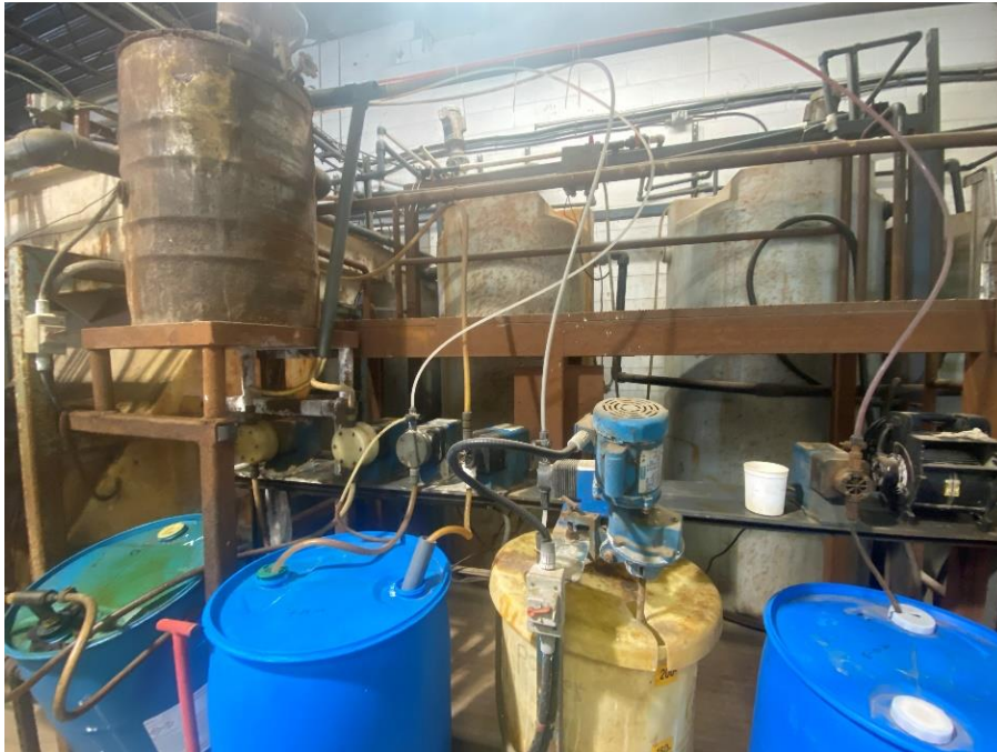
Figure 2-1: WWTP Clarifier and Separation Tanks
