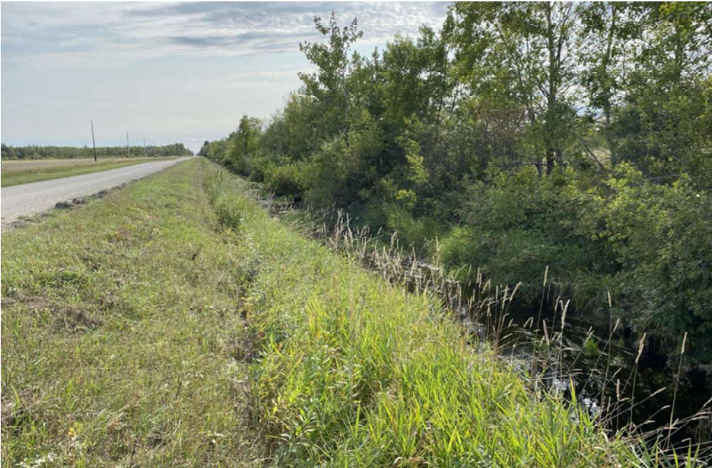
Photo No. 10: South Malonton Drain upstream of Rd 15N Access Crossing at STA 6+98 (looking upstream) – September 13, 2022
