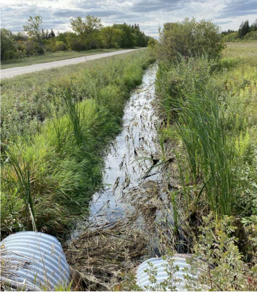
Photo No. 14: South Malonton Drain upstream of Rd 106N Access Crossing at STA 22+17 (looking upstream) – September 13, 2022
