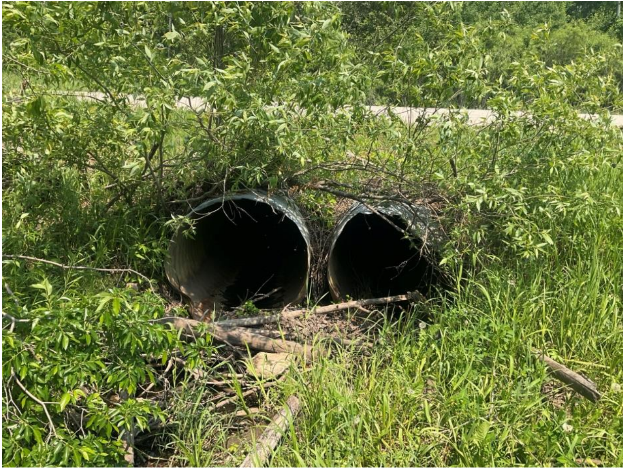
Photograph C-14. Looking downstream at WC-26 on the south side of the road. The culvert was partially blocked with debris, shallow standing water and no flow observed at the time of assessment (June 4, 2025).
