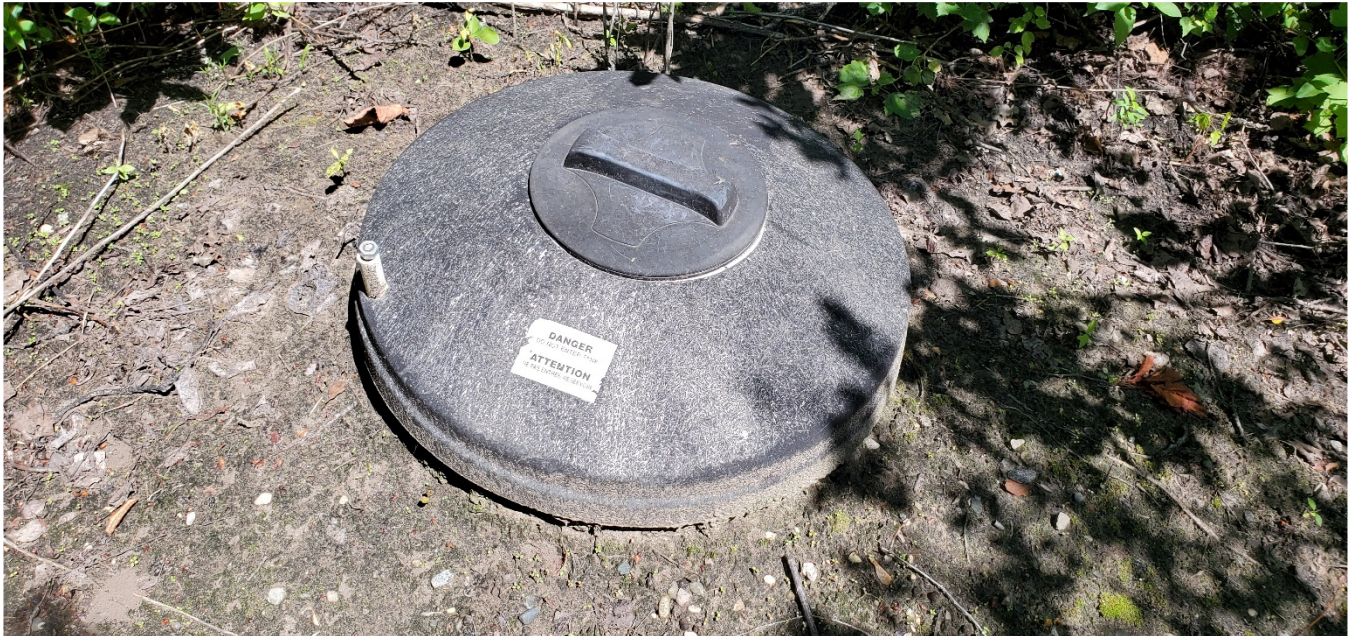
Photo A - RV Site Holding Tank
