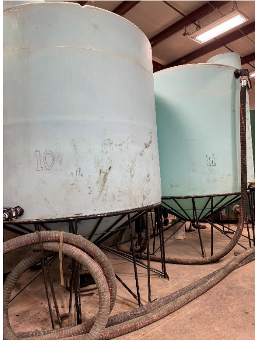
Photo 1 – View of the two new tanks in Building B at the Facility.
