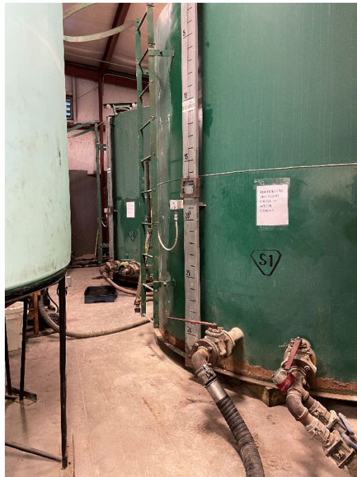
Photo 2 – View of some of the pre-existing tanks in Building B at the Facility.
