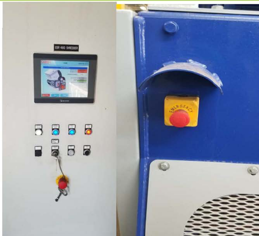
Location of both Emergency stops and the control panel
