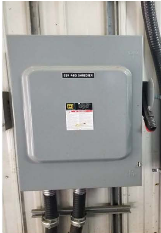
GSR 480 Main Power Switch
