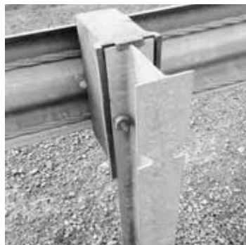
Figure 15. Bolt rail 1 and blockout to post 2.
