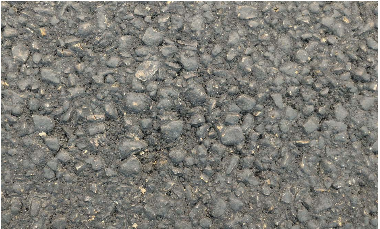
Figure 9 - Moderate (bordering on severe) Segregation
