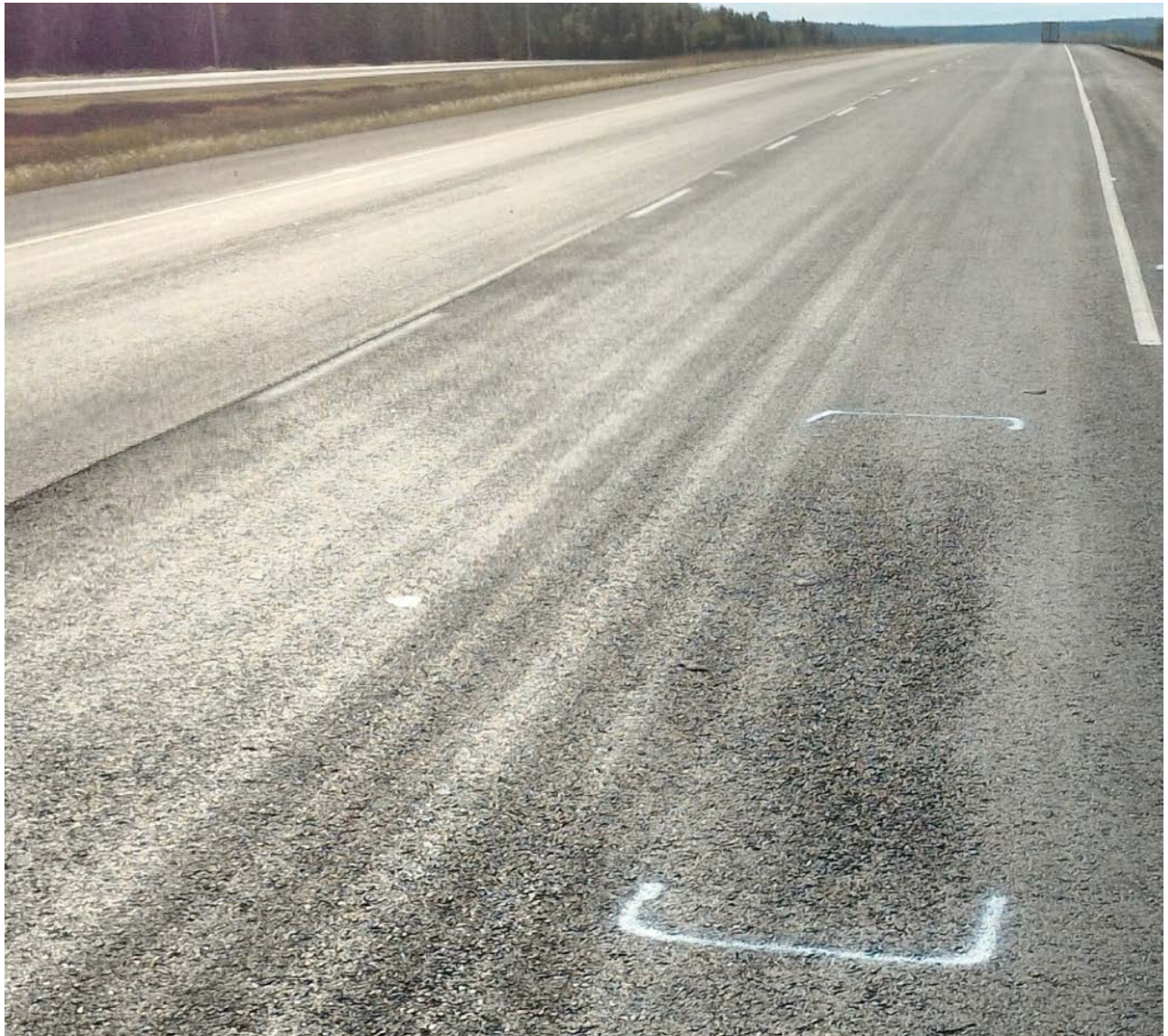
Figure 8 - Moderate (bordering on severe) Segregation
