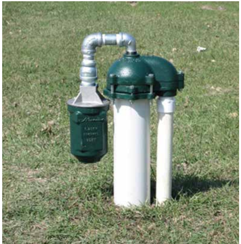
Flood protected well constructed with a watertight cap, snorkel well cap vent and cap cable seal
