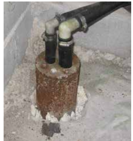
Sanitary well seal on a drilled well
