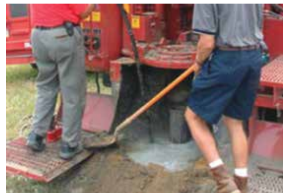
Placement of slurry grout using a tremie line (Photo credit – National Driller, August 2012)
