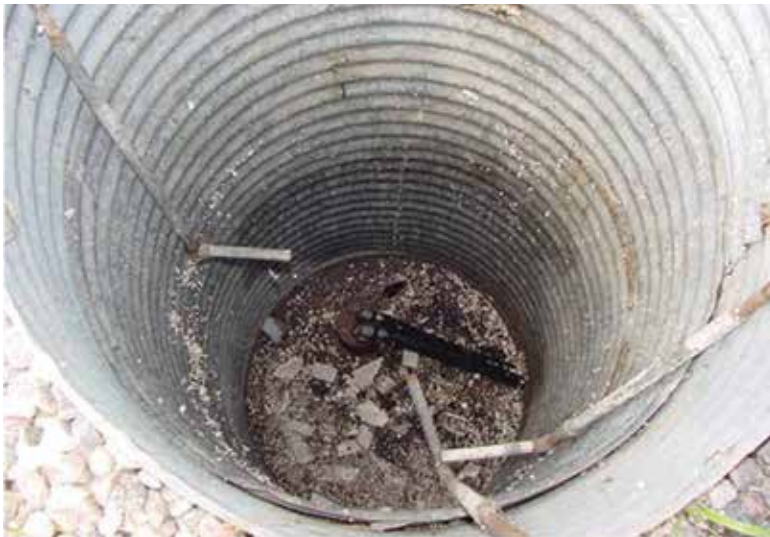
Well located inside of a well pit
