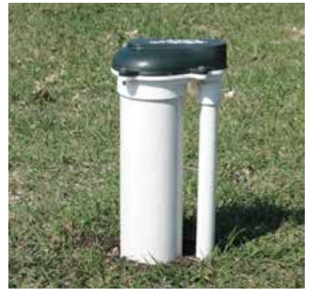
Well cap on a drilled well
